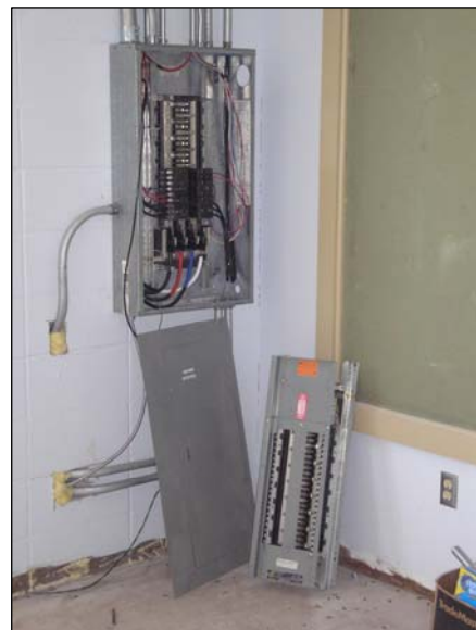
Electric panel and circuit breakers supply power to additional classroom equipment
