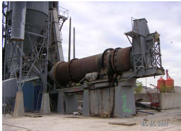
Asphalt plant rotary aggregate dryer and burner assembly
